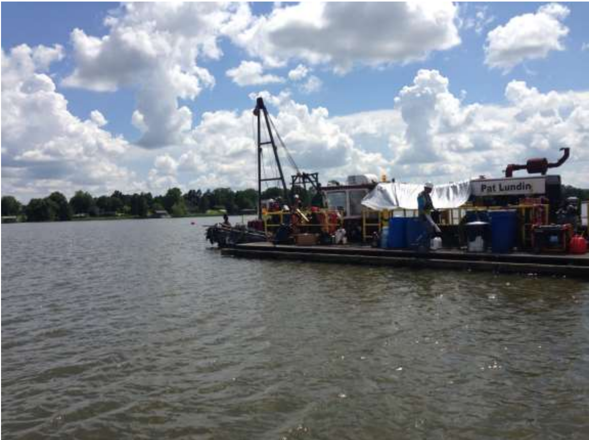
June 11, 2015 – View of the dredge while modifications are being made to the cutter head
